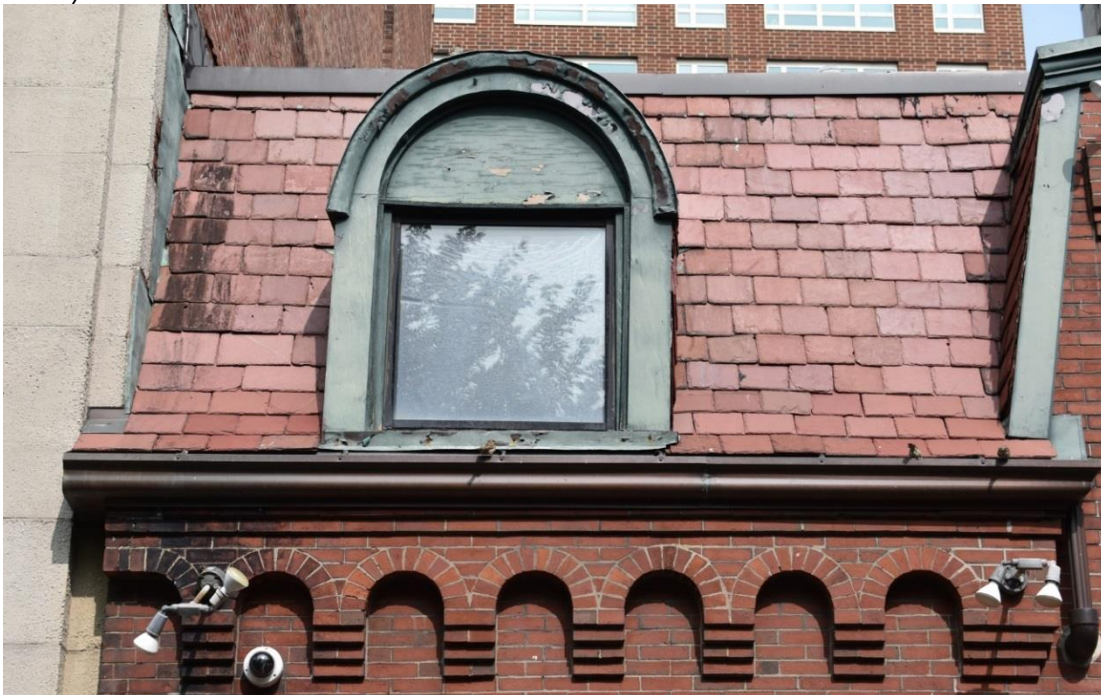
Photo 6. Detail of arched roof dormer, slate shingle Mansard roof, and corbeled cornice (west-half).
