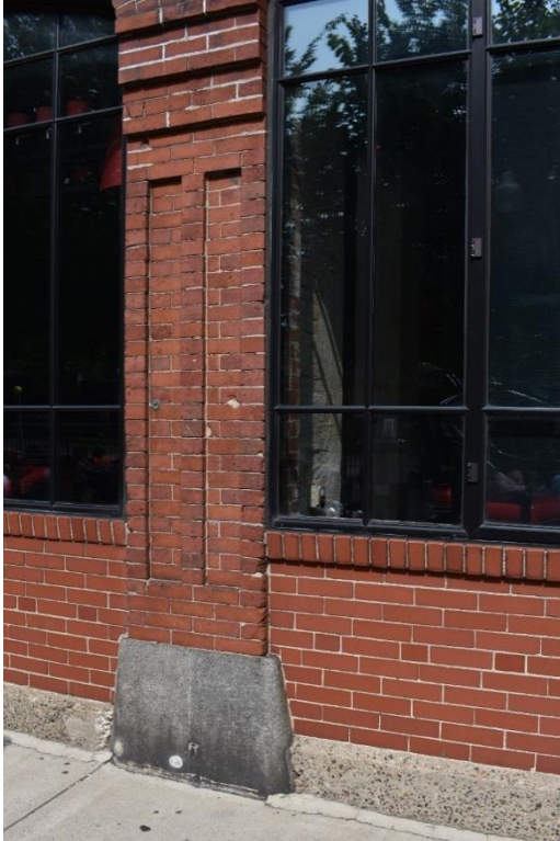
Photo 8. Detail of brick pilaster indicative of Panel Brick style and granite base blocks at carriage bays.
