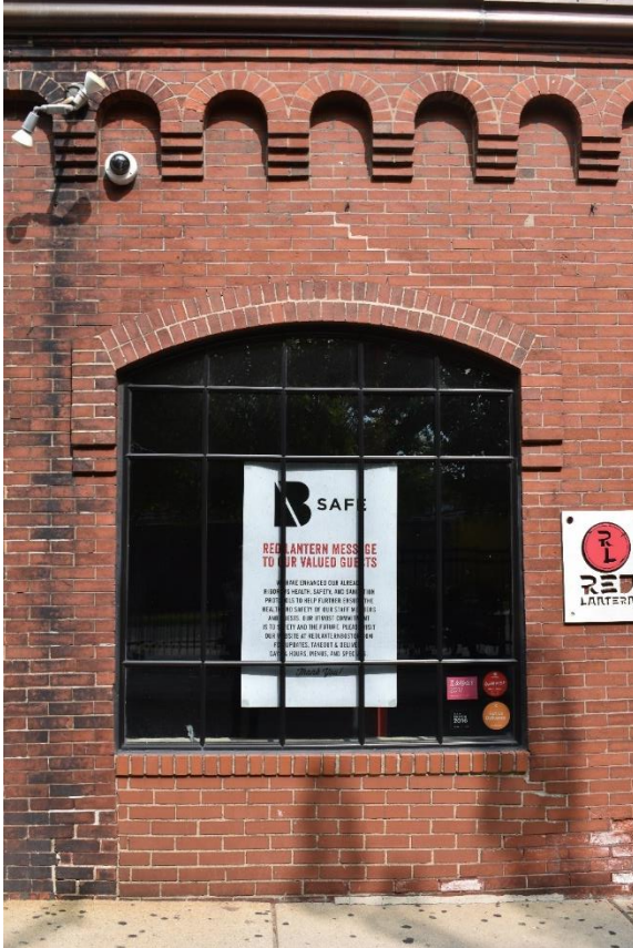
Photo 5. Window detail, west half of 39-45 Stanhope Street facade (first bay), looking north/northwest.
